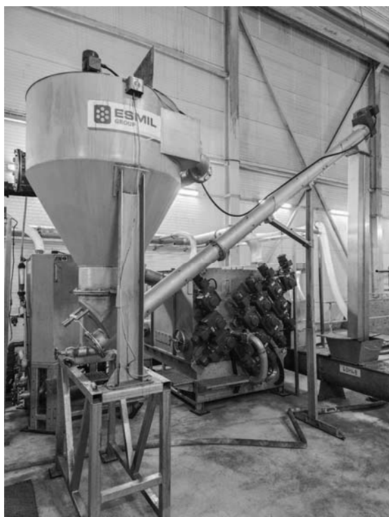
Figure 2 – Photo of the installation at the facility
