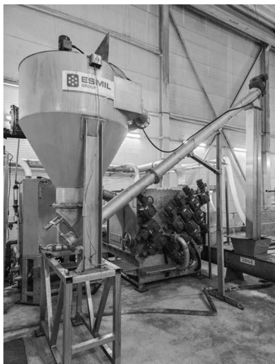
Figure 2 – Photo of the installation at the facility
